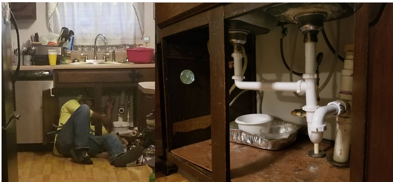
We repaired a leaking sink drain that would have caused this neighbor thousands in water damage.
